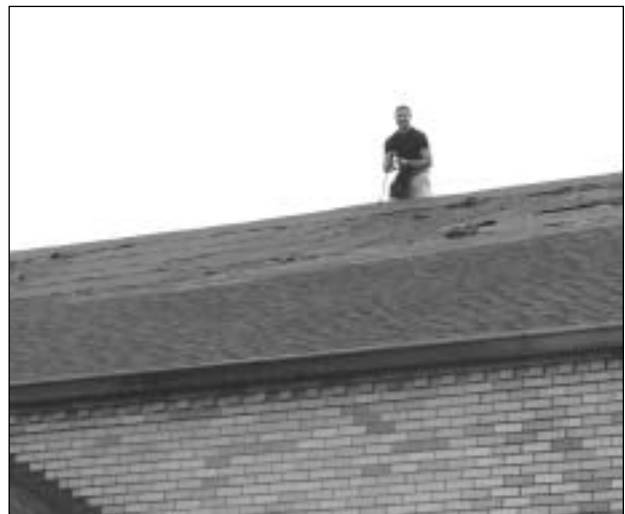
Fr. Michael Minifie working on the roof of Queen of Peace Church damaged by Hurricane Ike.
